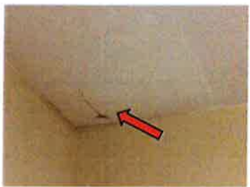
Photo 4 - Damage to ceiling drywall in living room area
