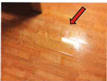
Photo 5 - Puddle of water forming on room floor
