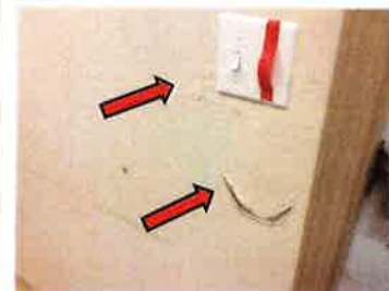
Photo 3 - Damage to interior drywall at east door
