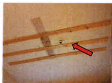
Photo 6 - Damage to ceiling drywall in shelter room
