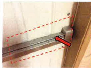
Photo 2 - Water accumulation along door exit mechanism
