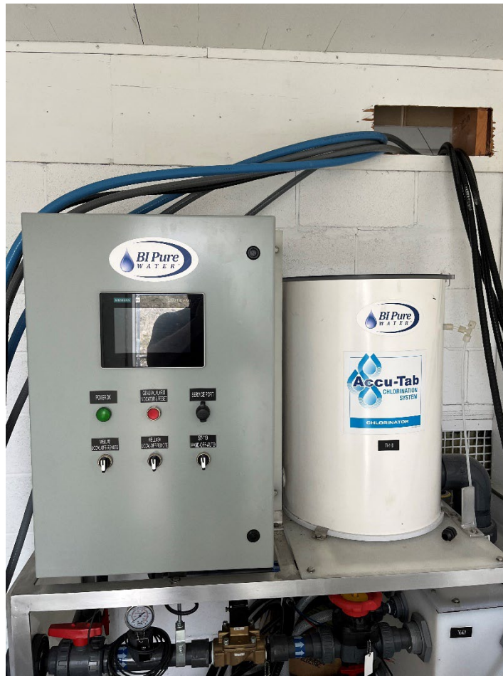
Figure 6: New Chlorinator Assembly for Well 3/3A.
