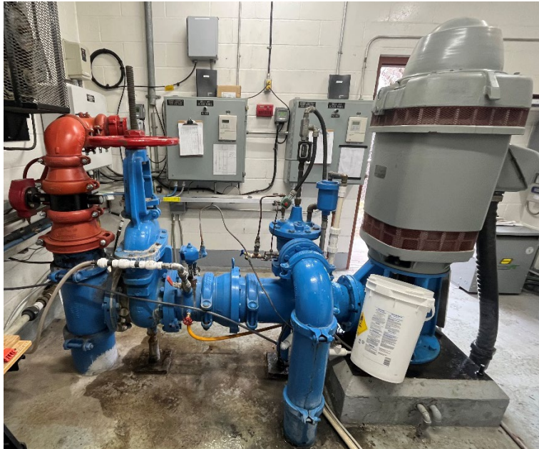
Figure 3: Well Pump and Piping to Water Distribution System.
