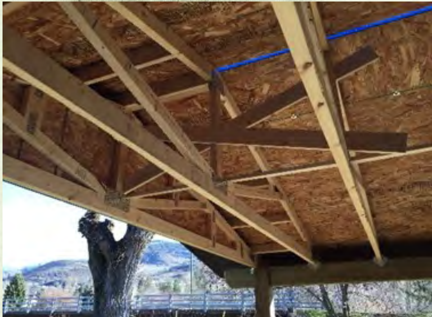
Roof Trusses with Hurricane Ties
