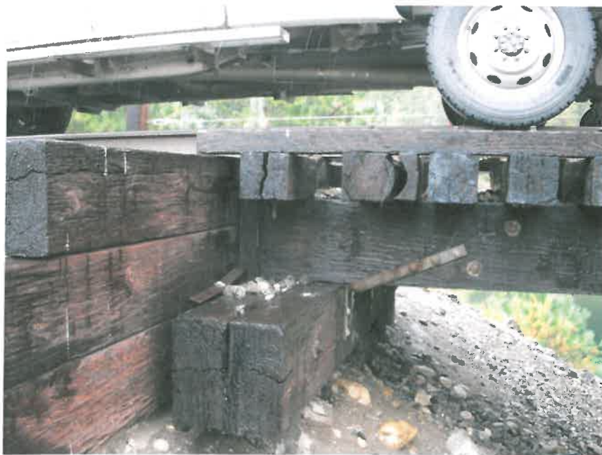
Mile 10.93 487' Combination Through Truss and Pile Trestle over the Kettle River Note failed bridge ties and splitting and rotating abutment sill
