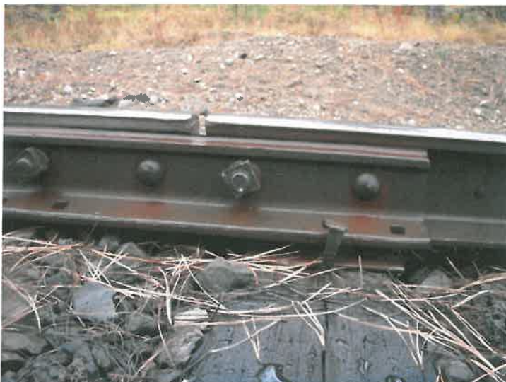
Typical low joint near Mile 19 Note that even good ties will not hold surface if the joint bars are loose Note: loose plate and 1" gap between the rail and tie plate A low joint results in more rapid tie deterioration due to impact.
